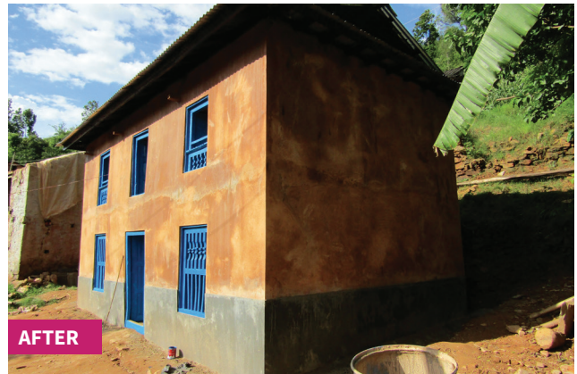
New ring beam, through ties, strongbacks, slab strips, plaster, stone gable infill replaced with lightweight timber panels, and improved roof 12
