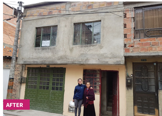
Added ring beam, confining elements, plaster and mesh plaster, upgraded roof, and improved sanitation
