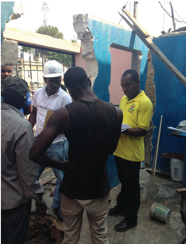
Engineer and building inspector reviewing the construction works with the builder, LAMIKA Housing Retrofit Project, Haiti, 2014.
