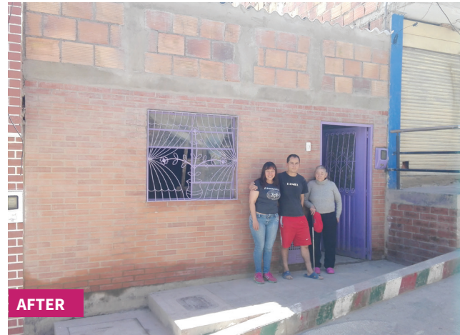
Added ring beam, confining elements, and plaster, and improved roof and sanitation
