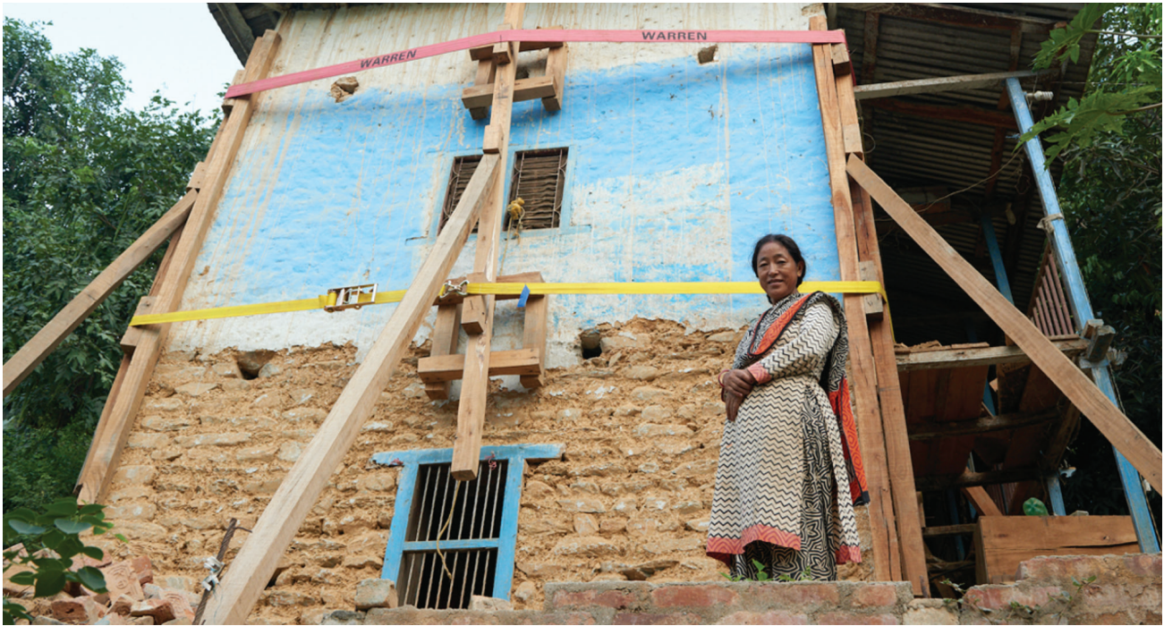
A homeowner in Nepal, where Build Change's technical innovation has enabled traditional rural homes to be retrofitted at national scale
