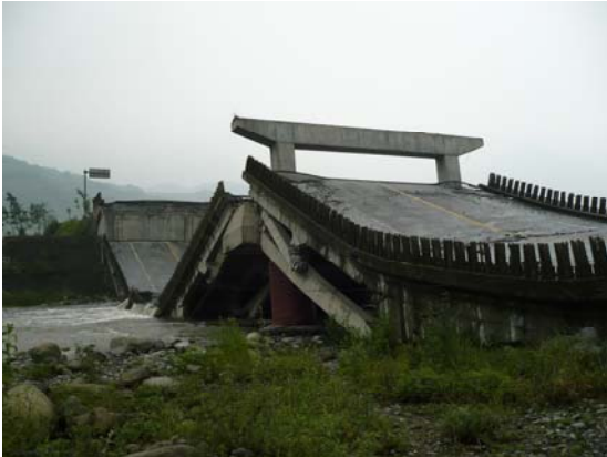
Fig 22. Collapsed 3 rd and 4 th spans. IMG0039
