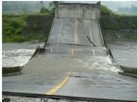
Fig 25. View of collapsed 4 th (westernmost) span, from 3 rd span. 4 th span displaced south relative to west approach. IMG0057
