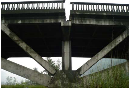
Fig 16. No damage to 2 nd span from the east (shown at left). IMG0032
