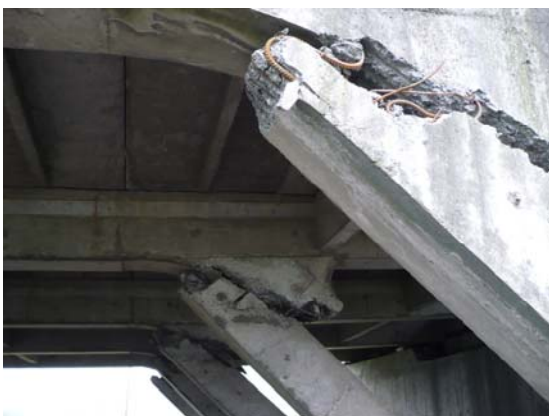
Fig 14. Spandrel element fractures. IMG0030
