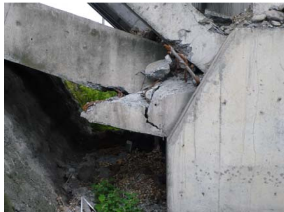
Fig 13. Fracture at connection between arch and abutment. IMG0019
