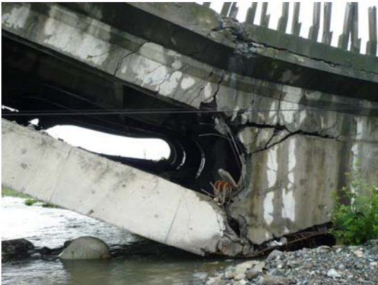
Fig 24. Damage at top of arch, 3 rd span. IMG0053
