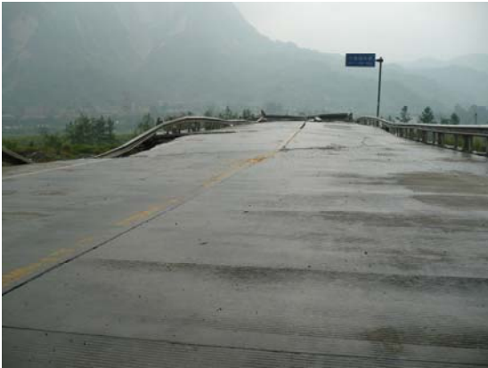
Fig 6. Heave in east bridge approach, looking west. Crack is consistent with NNW-trending ground scarp. IMG0012
