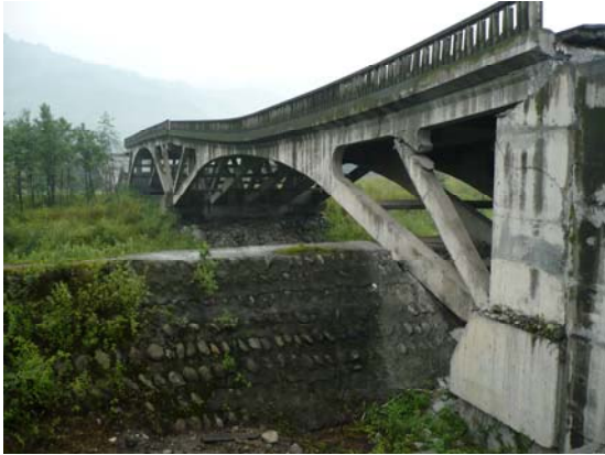
Fig 10. Easternmost span, east approach and abutment have moved west and/or arch has expanded due to fracture in RC elements. IMG0014
