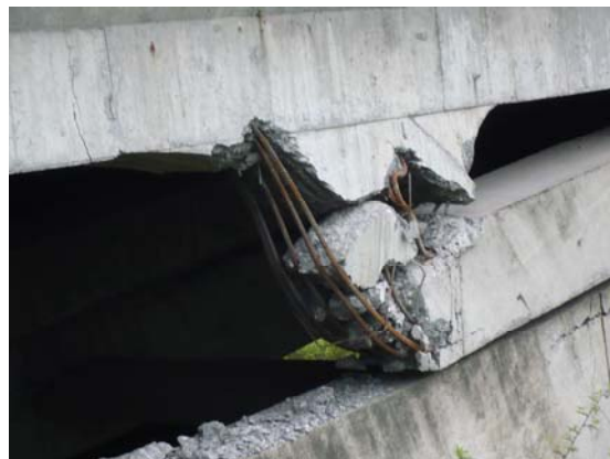
Fig 21. Fracture at spandrel connection, note lack of concrete confinement. IMG0041
