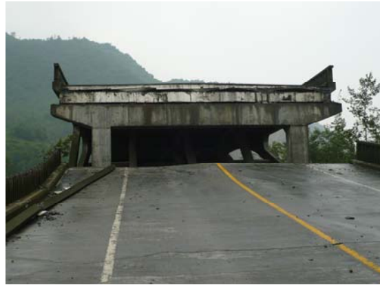
Fig 19. View from collapsed deck for 3 rd span, looking east at 2 nd span. 3 rd span appears to have shifted south. IMG0056
