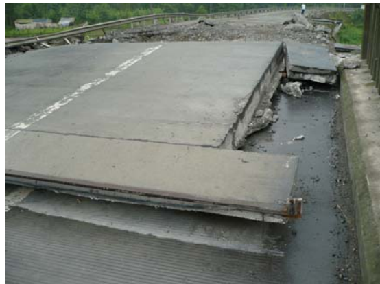
Fig 9. Displacement of road deck from east approach on top of first span, offset by over 3m west and twist to the north. Looking East. IMG0414
