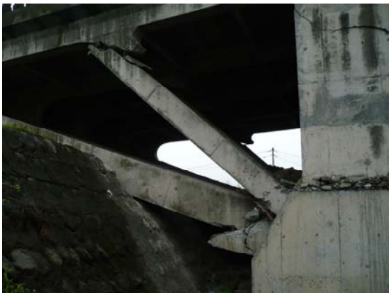
Fig 12. Fracture in spandrel elements. IMG0018
