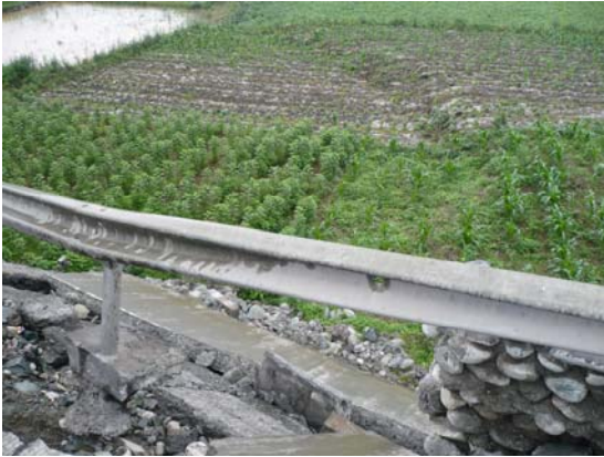
Fig 2. Permanent ground displacement, south side of bridge looking south, curved but trending NNW. West side moved up approximately 1.2m relative to east side. Possible extension to west. IMG0395
