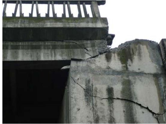
Fig 11. Relative displacement of east abutment and deck of easternmost span. IMG0020
