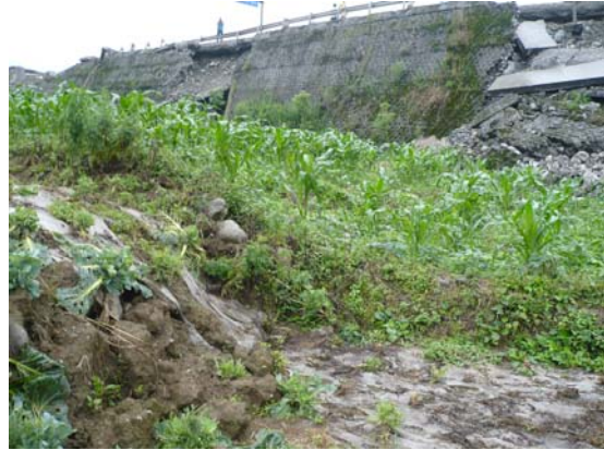
Fig 3. Permanent ground displacement, south side of bridge looking north-northwest, standing on the east (down block). West side moved up 1.2m relative to east side. IMG0404
