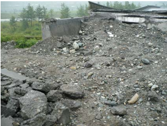
Fig 8. Collapse of road fill, east approach. Looking West. IMG0065
