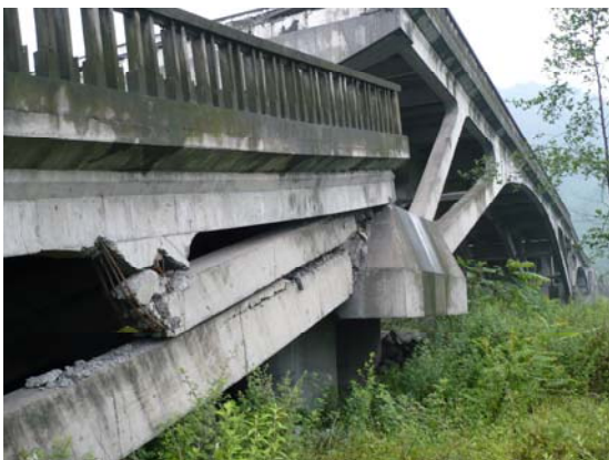
Fig 20. Collapsed deck and spandrel elements, 3 rd span looking east. IMG0040
