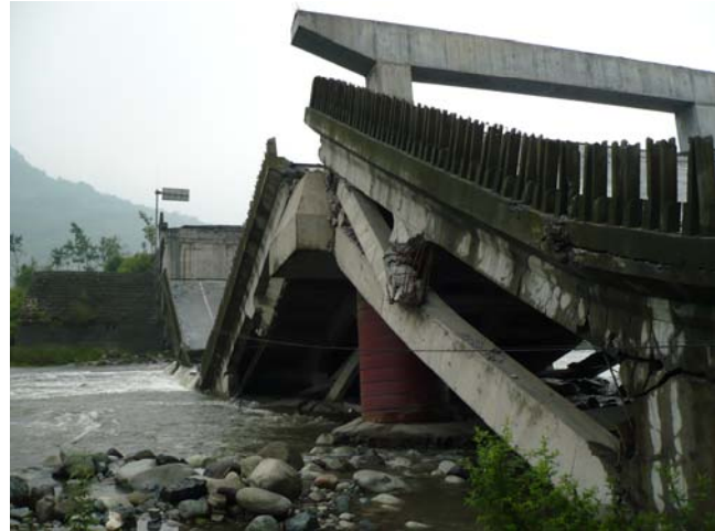
Fig 1. Collapsed westernmost spans of four-span, reinforced concrete arch bridge at Xiao Yu Dong. IMG0047.
