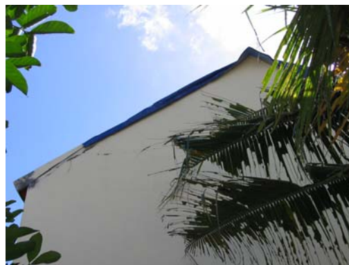
Figure 12. Crack at masonry gable, CEEDEDS house, Jejeran-2, Wonokromo, Pleret (Bantul), S7.86676° E110.38764°, IMG_6696
