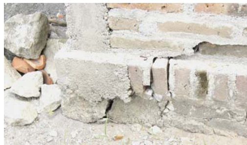
Figure 28. Sliding along wall/foundation interface, Tegal Kebong Agung, Imogiri (Bantul) S7.93434° E110.36667°, CIMG1769
