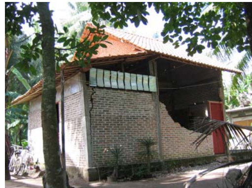
Figure 23. Collapse of masonry wall (note absence of ring beam), Kebutren, Pleret (Bantul) S7.86905° E110.40272°, IMG_6725
