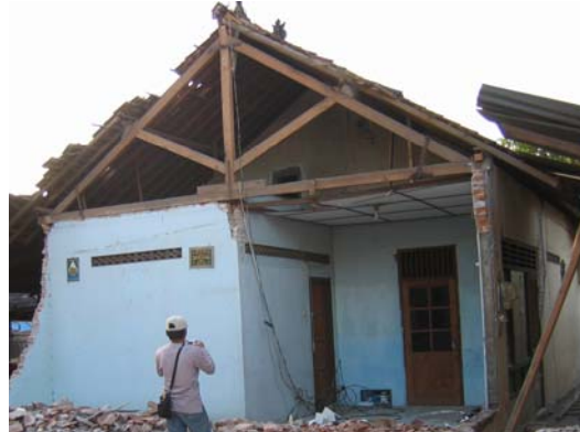
Figure 25. Typical timber truss with steel plates reinforcing the joints, Kasongan, Kasihan (Bantul), S7.84512° E110.33534° IMG_6831.
