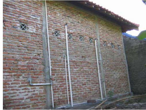
Figure 9. Backside of well designed and built confined brick masonry house, Bebekan Mulyodadi, Bambang Lipuro (Bantul), S7.94160°, E110.32297°, IMG_6804
