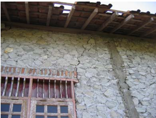
Figure 10. Partially confined stone masonry house with timber ring beam, Platar Somopuro, Jokonalan (Klaten), S7.75478, E110.53557, IMG_6897
