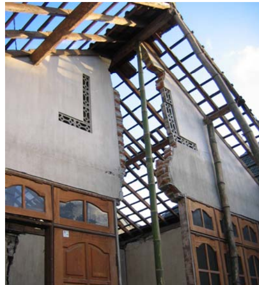
Figure 21. Collapse of offset gable, Kasongan, Kasihan (Bantul), S7.84512° E110.33534°, IMG_6824
