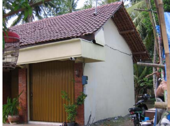
Figure 19. Masonry gable wall overturning (Bantul) S7.89468°, E110.37341°, IMG_6542
