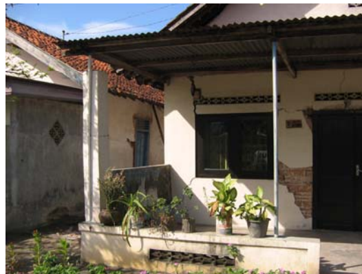
Figure 5. Unreinforced masonry house, damage category D3, Tlogo, Prambanan (Klaten), S7.75259° E110.49550° IMG_6852
