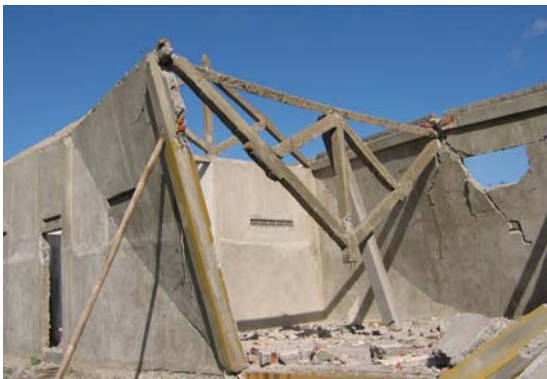
Figure 26. House/shop with reinforced concrete truss, Bebekan Mulyodadi, Bambang Lipuro (Bantul) S7.93460° E110.32194°, IMG_6778
