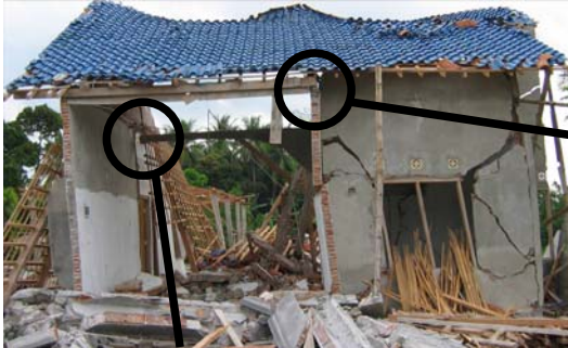
Figure 13. Confined masonry house under construction, insufficient connections, Pleret (Bantul). S7.87574°, E110.40703°, IMG_6575
