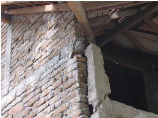
Figure 17. Insufficient connection between column and beam, Pleret (Bantul) S7.88174° E100.40869°, IMG_6746
