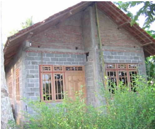
Figure 20. Minor damage to offset gable, Gantiwarno (Klaten), S7.75485° E110.53555°, IMG_6905
