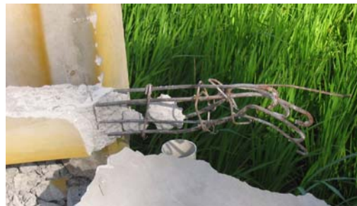
Figure 27. Reinforcement in beam for house/shop, Bebekan Mulyodadi, Bambang Lipuro (Bantul) S7.93460° E110.32194°, IMG_6781
