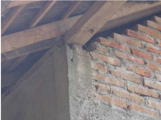
Figure 24. Common connection between column and beam – column steel wrapped around timber, Jejeran-1, Wonokromo, Pleret (Bantul), S7.86480° E110.38821° IMG_6672.
