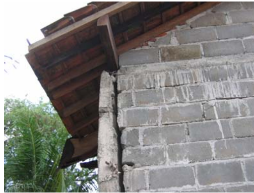
Figure 16. Insufficient connection between column and beam, Segoroyoso, Pleret (Bantul) S7.88174° E100.40869°, IMG_6749
