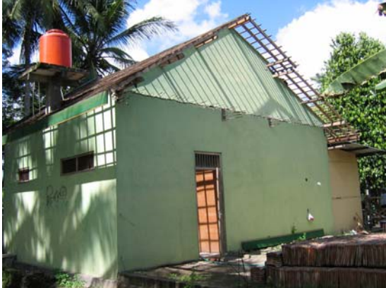
Figure 18. Masonry gable wall overturning, Keputren, Pleret (Bantul) S7.86905° E110.40272°, IMG_6721
